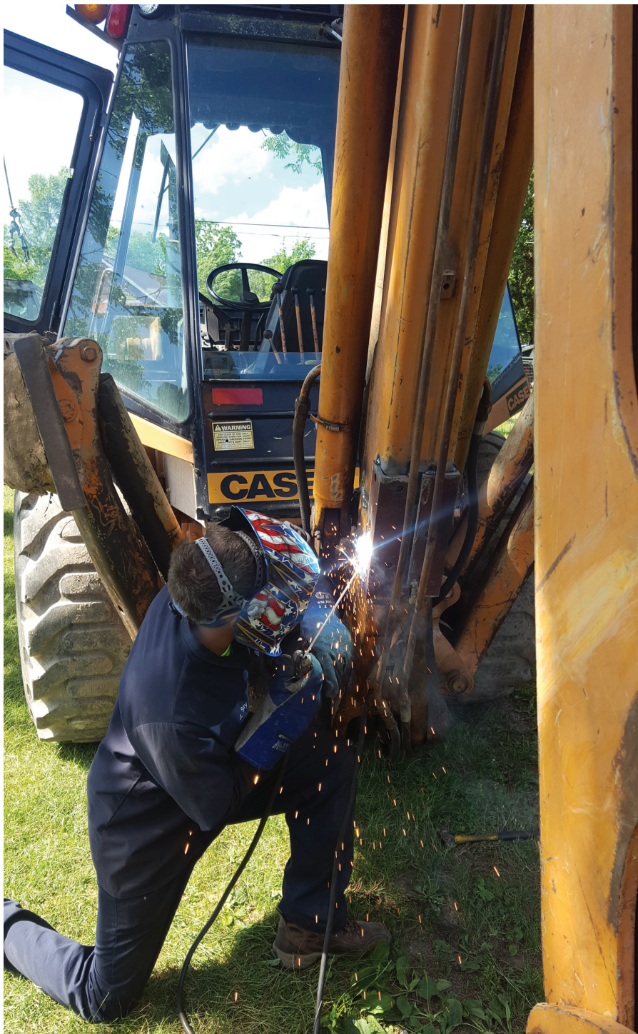
Fig. 2 — Sly on an emergency call; the arm on this backhoe loader split and needed immediate repairs.
